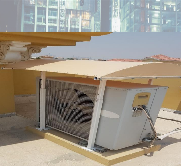
GENERATOR COVER - VILLA
